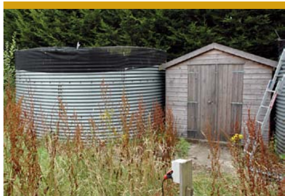
Borehole pump & water tank
